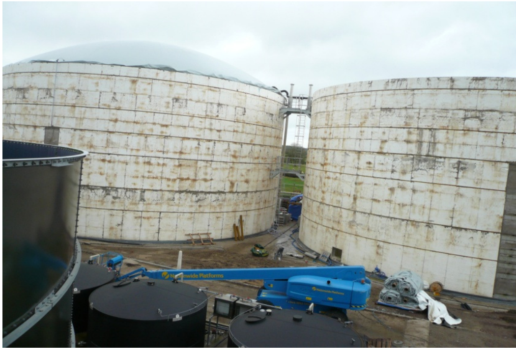
Image 1 – On-site AD and Gas to Grid Plant at First Milk, Aspatria
