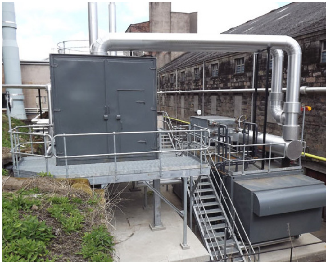
Image 2 - On site CHP and Boiler Installation to Maximise Revenue
